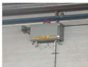
Current indicator light for LVL Hydraulic room is RED . Should be CLEAR to indicate severe upset Requires immediate attention.
