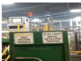
Current indicator lights on Hog System. BLUE for Metal Detector. AMBER for Hog System Trouble. Should be changed to GREEN for Metal Detector. CLEAR for Hog System Trouble
