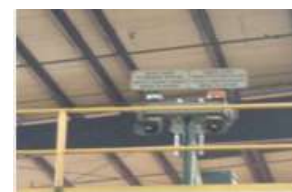
Current indicator light for RTO is BLUE and current indicator light for spark detection is ORANGE . Should be Green for RTO upset and CLEAR for Spark detection immediate attention.
