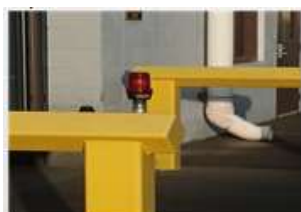
Roll up door cross walk next to maintenance. Current indicator light is RED . Should be BLUE for Hyster Pedestrian Interaction.
