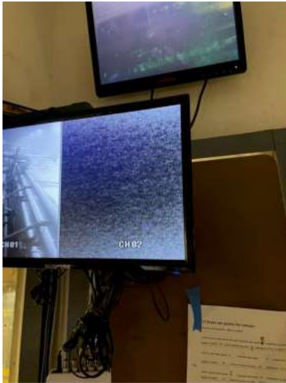
Camera Feed to Dryer Shack, White Hot indicates Fire/sparks
