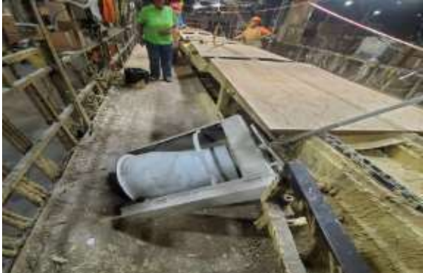
Sonic Air Fan Fell from Ceiling
