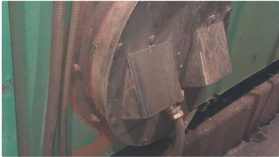
System installed on the Dryers
