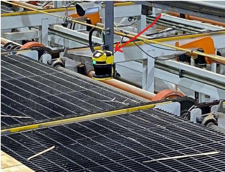
One of (2) 270 degree LOTO safety lasers mounted 6 inches from the grating
