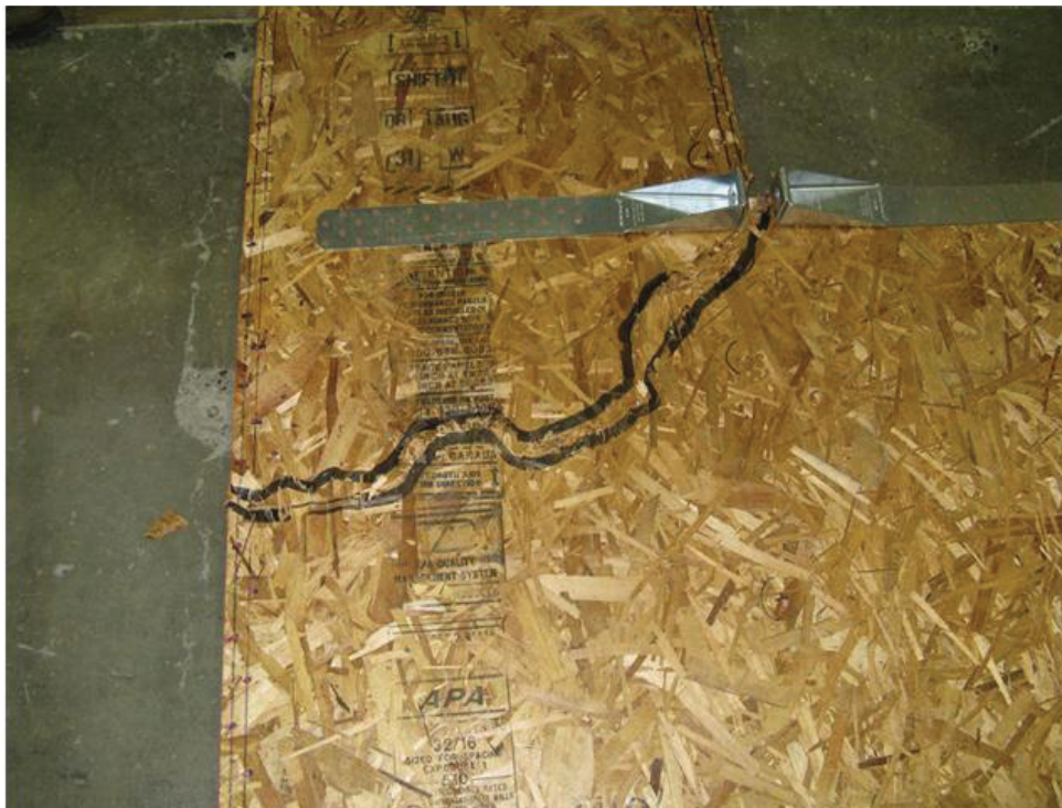
WALL 6A, SHEATHING TEARING, BOTTOM EAST STRAP
