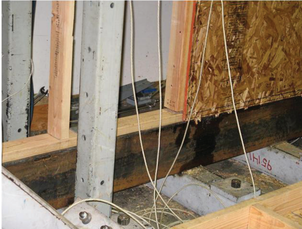
WALL 7B, NAIL HEAD PULL-OUT FROM BOTTOM OF PANEL
