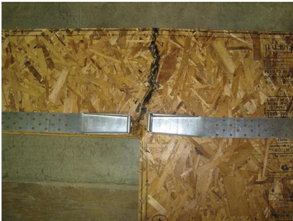
WALL 6A, SHEATHING TEARING, TOP WEST STRAP
