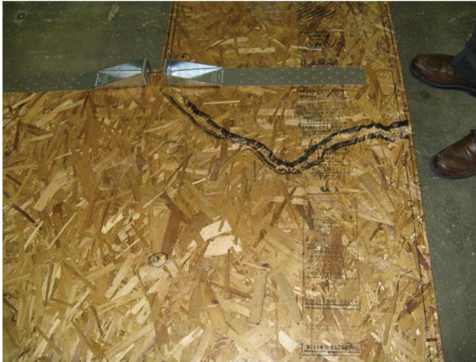
WALL 6A, SHEATHING TEARING, BOTTOM WEST STRAP
