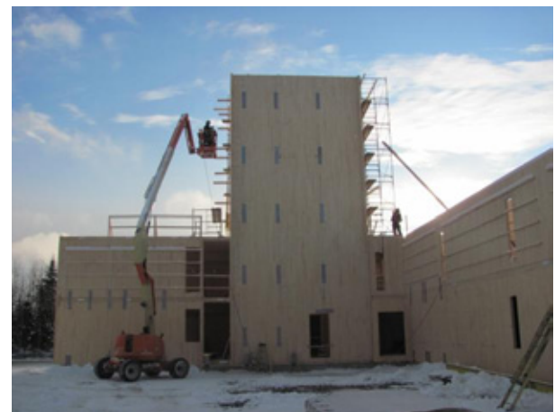
Figure 3: A 4-story CLT apartment building under construction in Quebec, Canada (photo courtesy of Nordic Engineered Wood, Chibougamau, Quebec, Canada)
