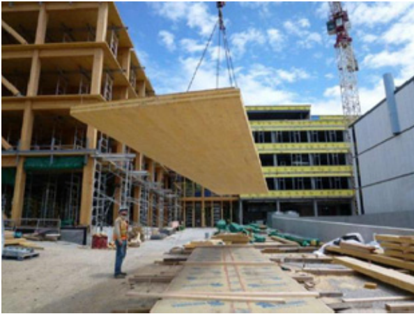
Figure 4: The Earth Science Building at the University of British Columbia under construction in British Columbia, Canada (photo courtesy of Structurlam, Penticton, BC, Canada)
