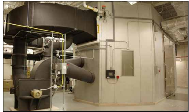
Figure 3. FPL's Chamber for Analytic Research on Wall Assemblies exposed to Simulated weather (CARWASH). Photo by Steve Schmieding
