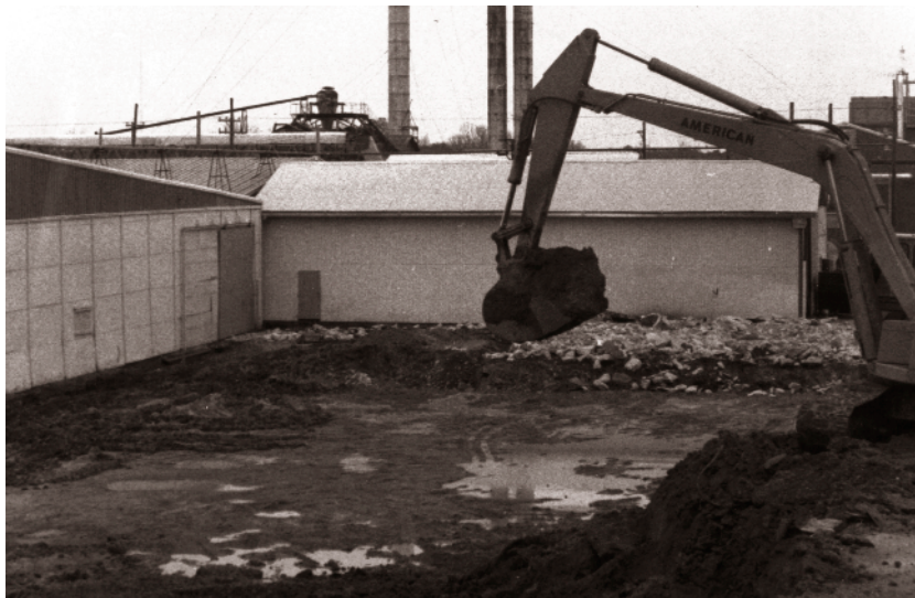
Construction sequences from the 1976 expansion of the plant's facilities, nearly doubling capacity.
