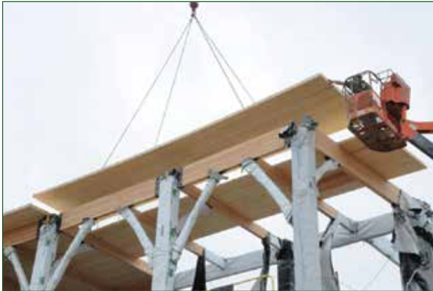
CLT roof panel being lifted into place at the new Promega Corporation facility.
