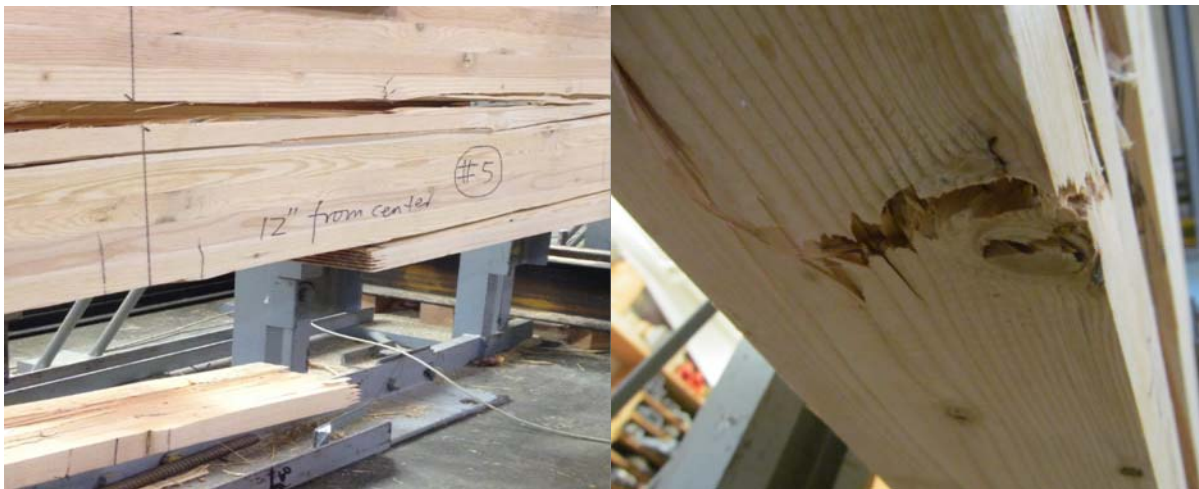
Figure 4. Glulam beam failure modes
