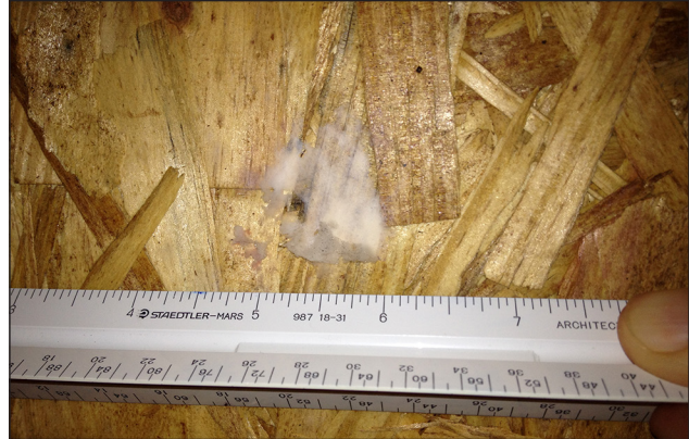
Mold growth on oriented strandboard sheathing.
