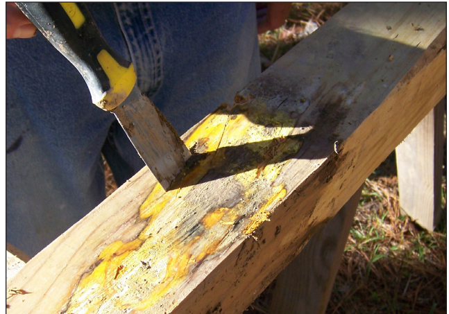
Figure 1. Damage caused by a copper-tolerant fungus growing on a wooden post treated with a copper-based preservative.
