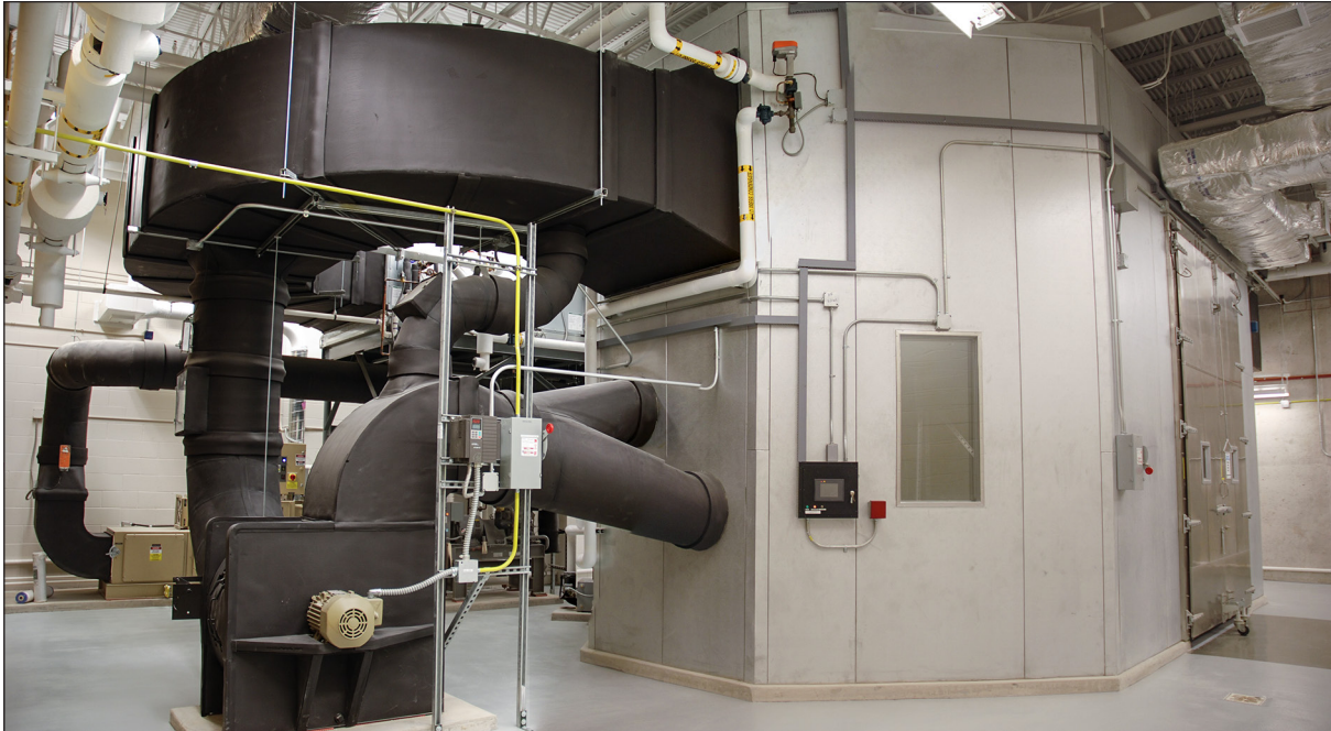
Figure 2—Chamber for Analytic Research on Wall Assemblies exposed to Simulated weather (CARWASH) facility [credit: Steve Schmieding].
