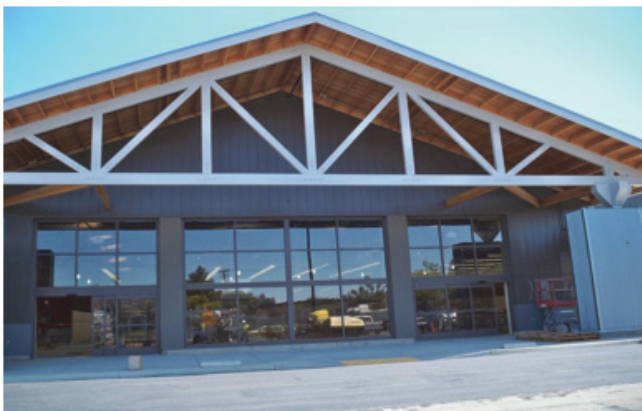
Figure 20: Partially Exposed Glued-laminated Timber Truss
