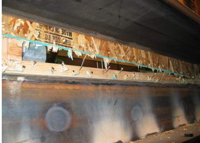
Figure 5. Typical failure mode from uplift only tests (Wall A2)
