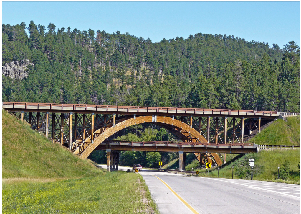
Timber bridges located between highways US16 and US16A in Pennington County, South Dakota: Timber Girder Bridge and Keystone Wye Timber Arch Bridge.
